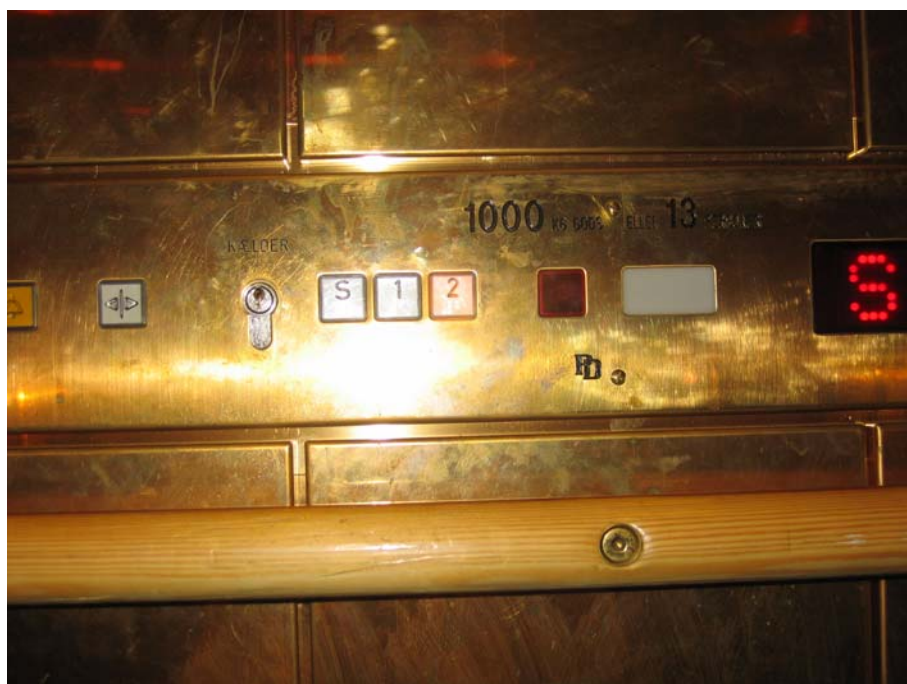
Illustration 9. Betjeningspanel i elevator
